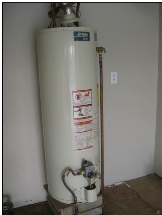
32. Service water heater
