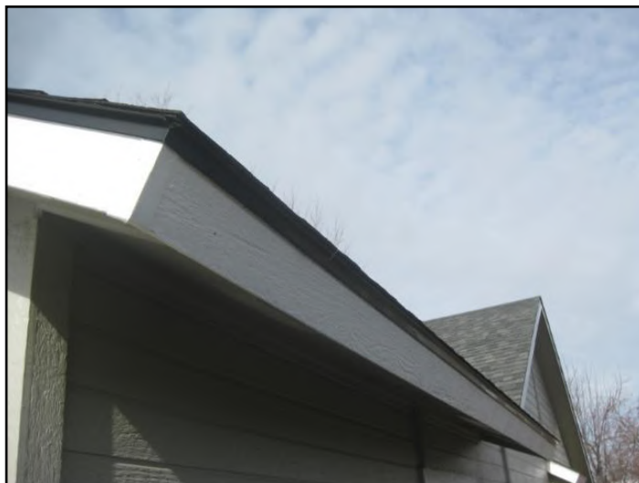
12. Recommend gutters and downspouts around the...
