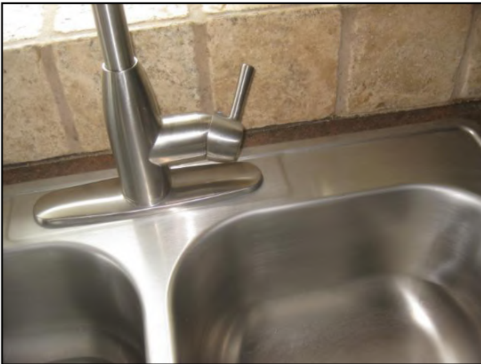
46. Backflow prevention missing
