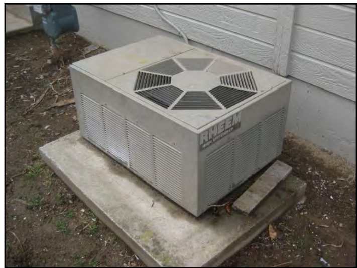
27. Recommend servicing AC unit(s) annually.
