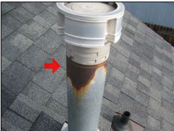
22. Rust at B vent
